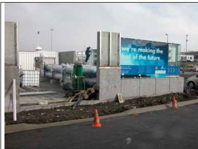
Fig 5 the construction of the auxiliary parts of the hydrogen station. The ready made components are all in place.
