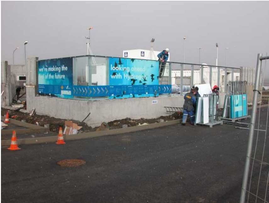
Fig 3. The impressive external design of the first hydrogen fuel station in Reykjavik does not reveal all its splendid safety features.
